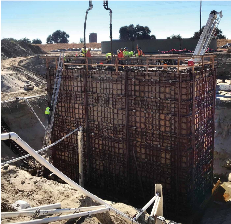
River Island Sewage Pump Station, California, USA Pump/Lift Station • Xypex Bio-San C500
